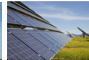
Solar panels. Spain.
